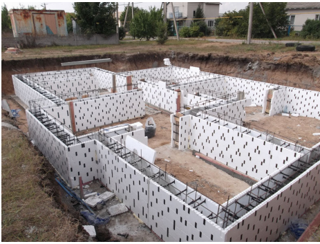
The foundation of the new Coworker and Bible School building at Petrodolina
